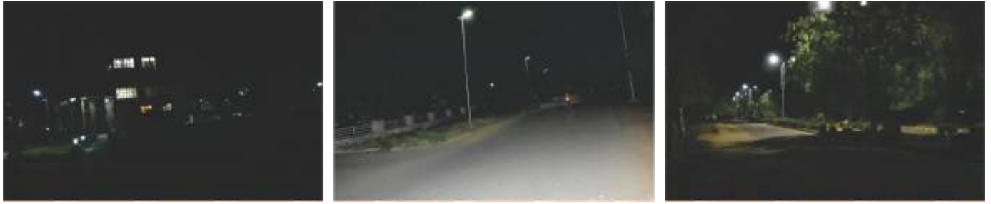
Solar street light at the New and Old Campuses
